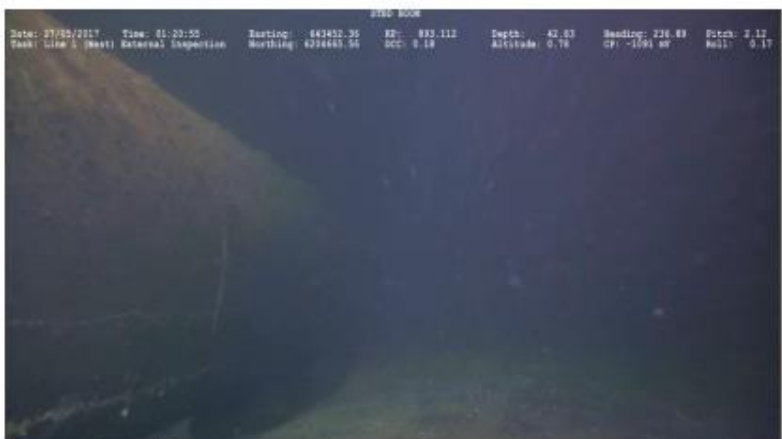
Boom camera too far out
